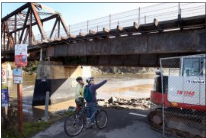
Cyclists pause at the San Lorenzo River Trestle Bridge, where work has begun to widen the pedestrian walkway.
