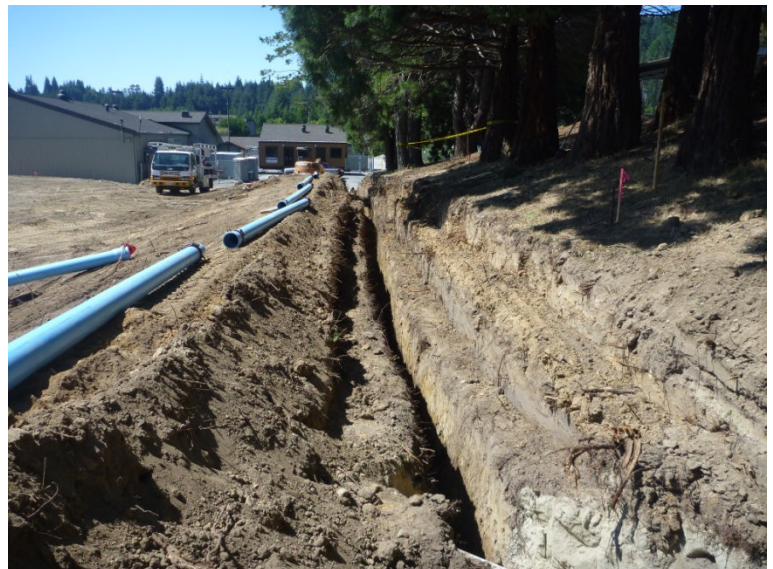
Image above shows a 6" Fire Service water trench relocated to allow creation of a plaza at the entrance to the new library
